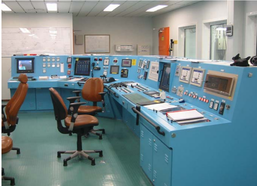
Figure 6. Cargo ship engine control room
