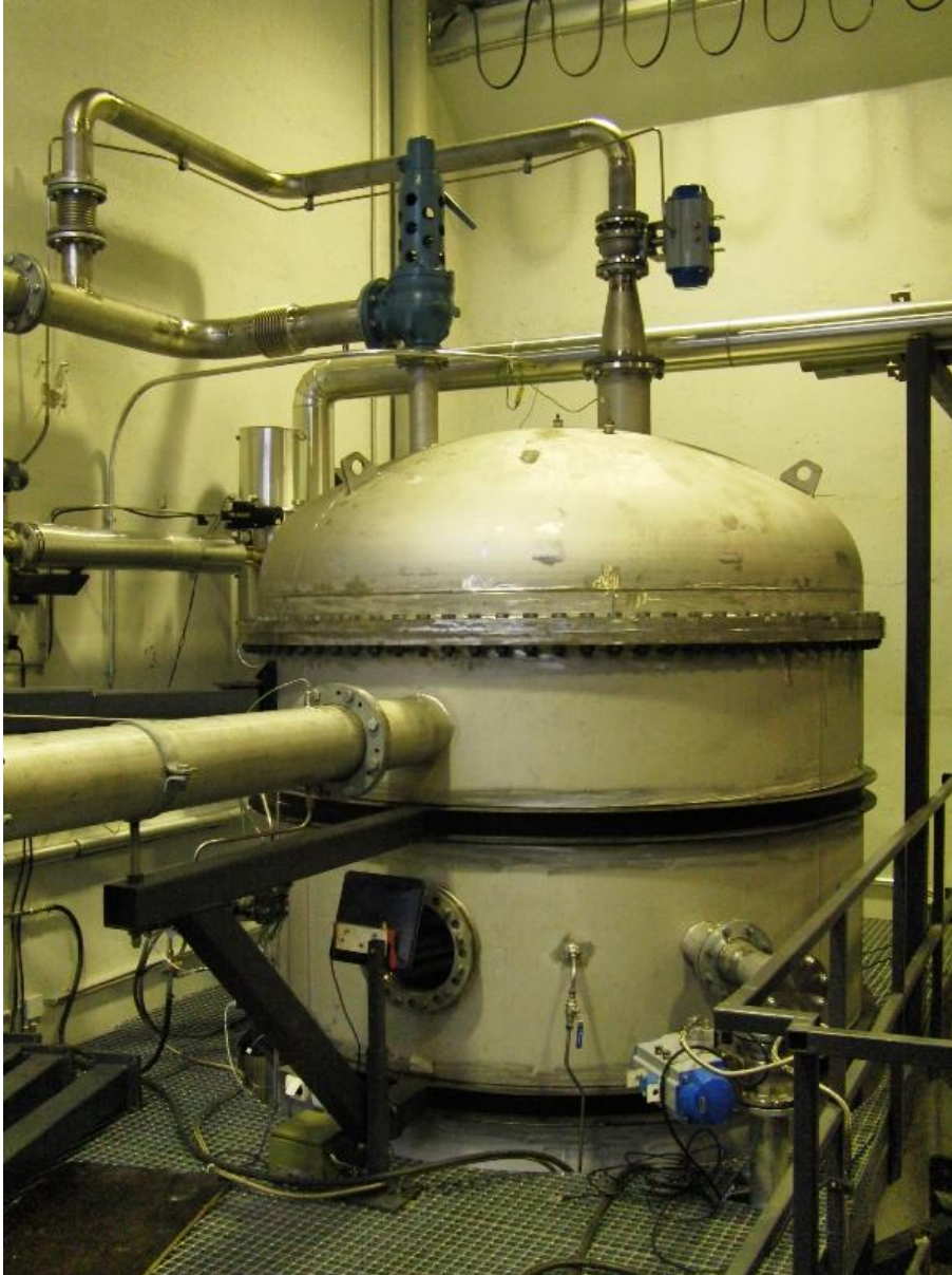
Dry well compartment, relief valves and inlet plenum.
