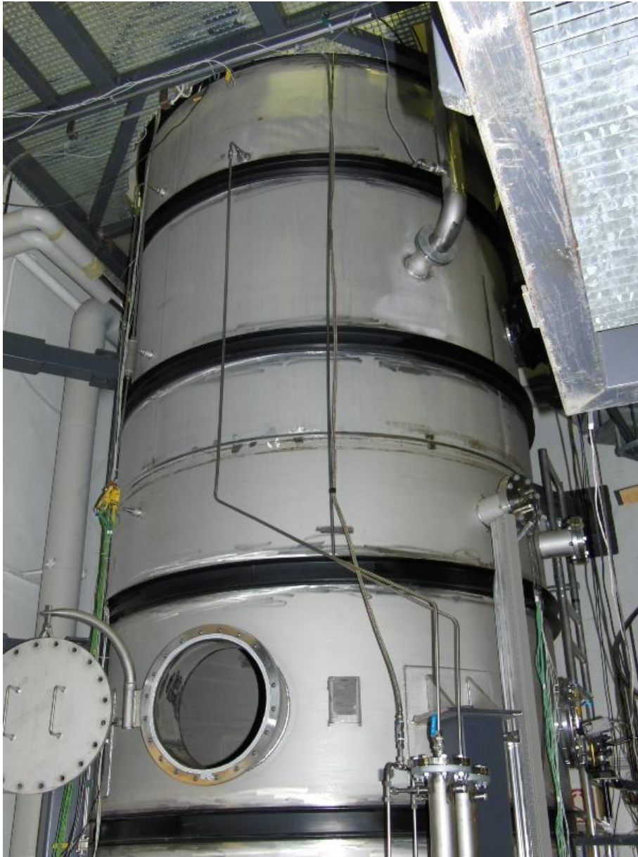
Piping system for condensate collection tanks 3 and 4.
