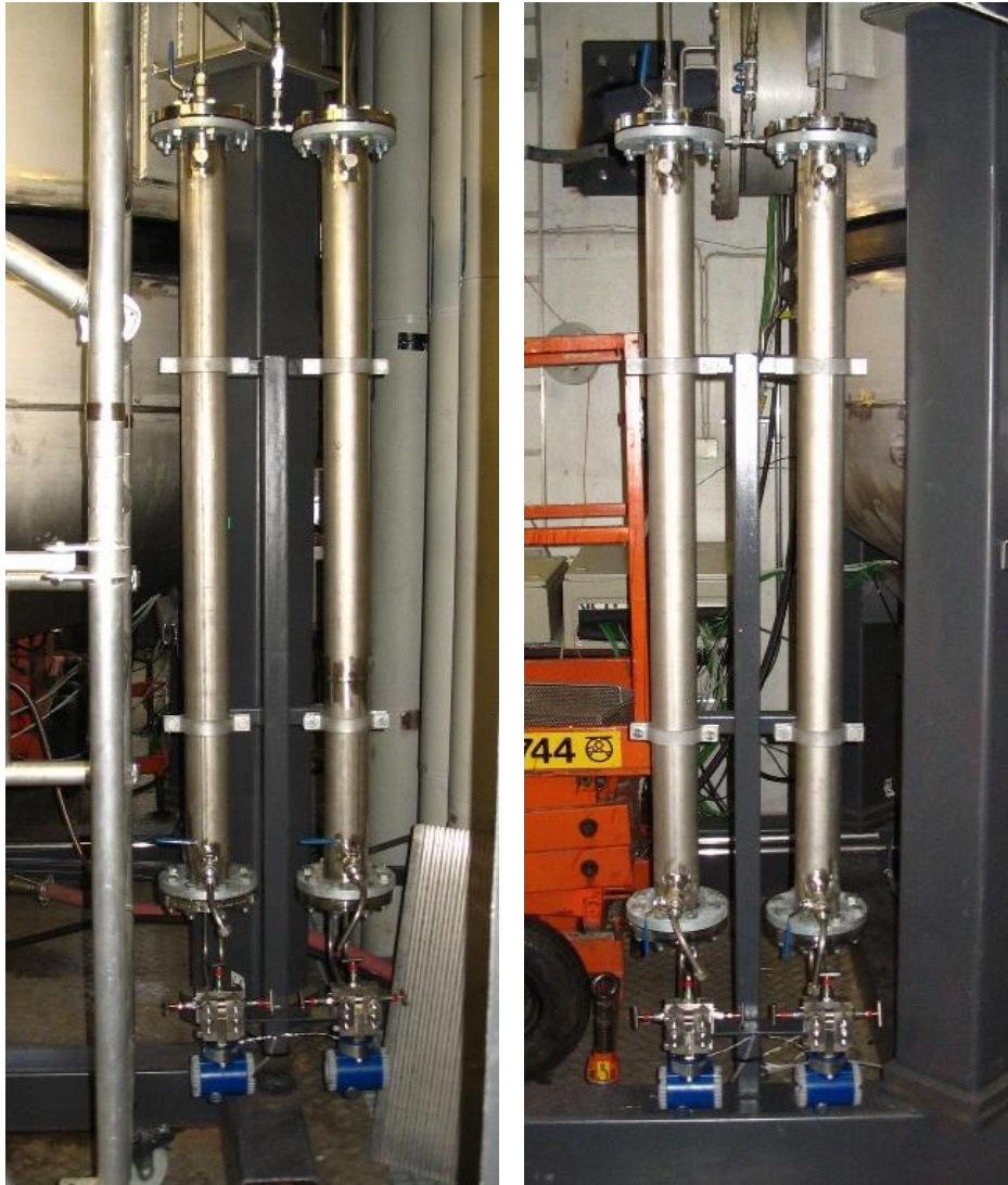
Condensate collection tanks 1 and 2 (left) and tanks 3 and 4 (right).
