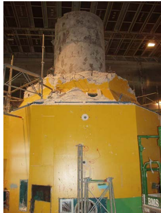
Figure 15 Chimney down, reactor tank exposed
