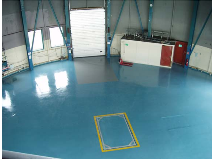
Figure 17 The floor in the reactor building after removal of the reactor. The hole in the floor has been closed by a removable lid, giving access to the basement.
