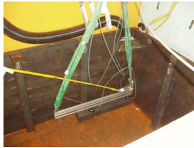
Figure 7 Graphite stringers removed and placed in waste container by use of vacuum lifting device
